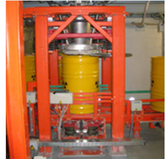
Drum Filling Station
