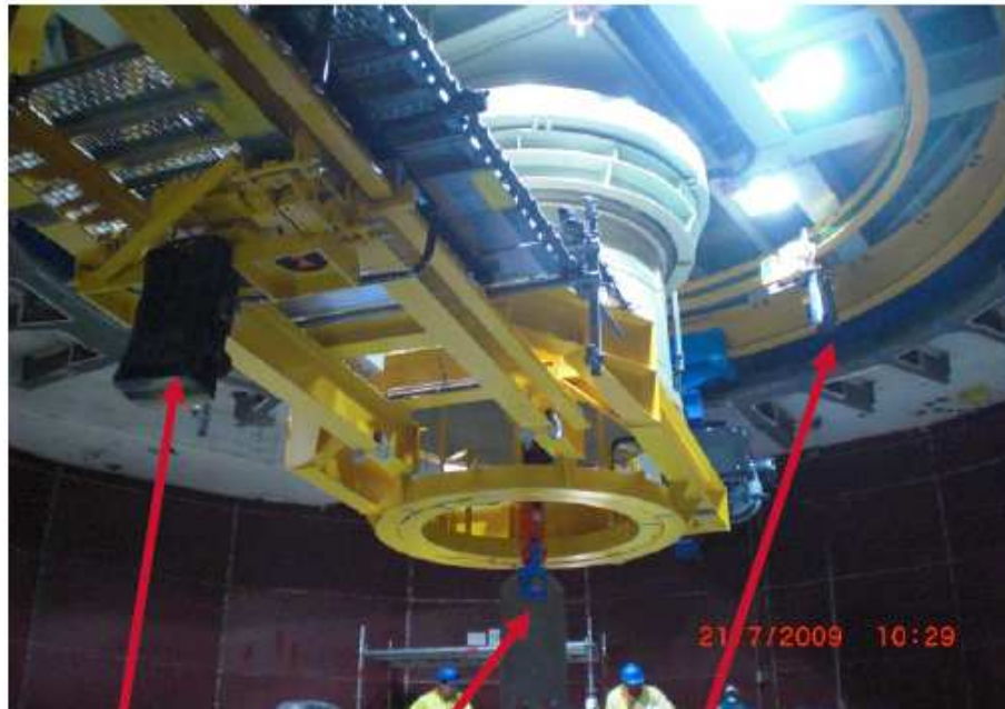
2t lifting unit
